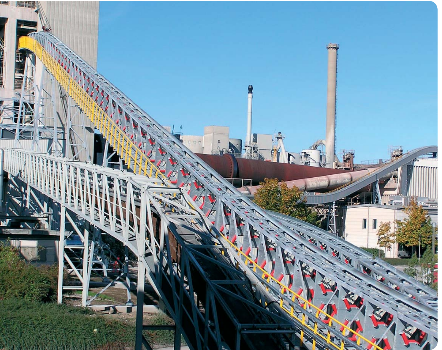
Construction of new conveyor and feed installation for supply of alternative fuel to Kiln 87
