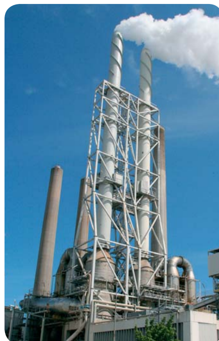
Installation for recovery and supply of waste heat for district heating
