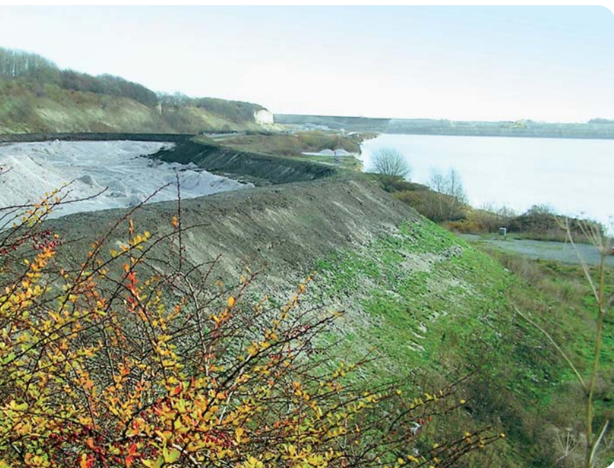
Use of microfiller in construction of embankment as part of chalk pit rehabilitation
