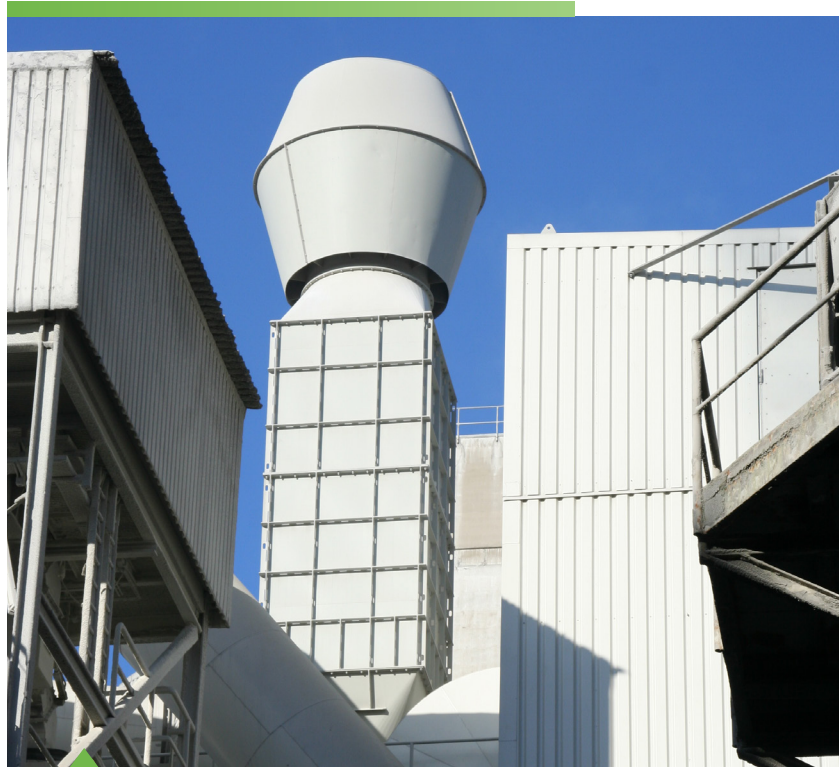
CEMENT MILL 4 UPGRADED TO CIRCULATION MILL WITH SEPARATOR
